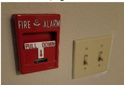
Alarm Points/Light Switches
